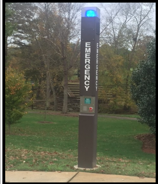
Campus Emergency Phone (Stanchion)
