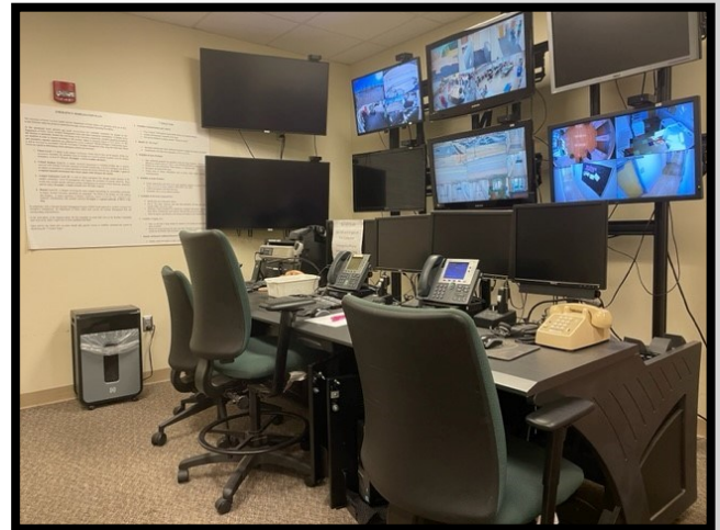
CCTV Monitoring Room
